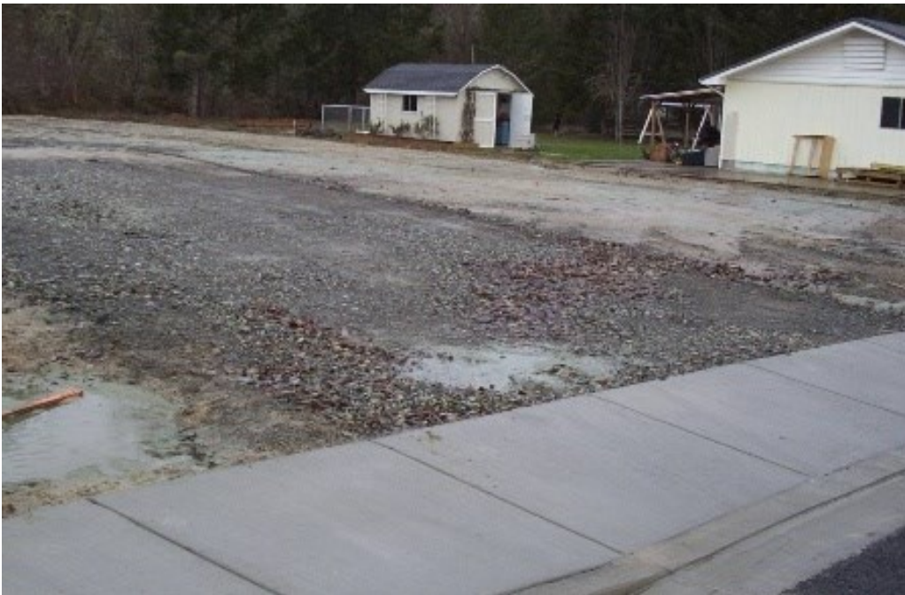
Temporary construction entrances (left) help keep debris onsite and can provide a suitable subbase for future driveway paving.
