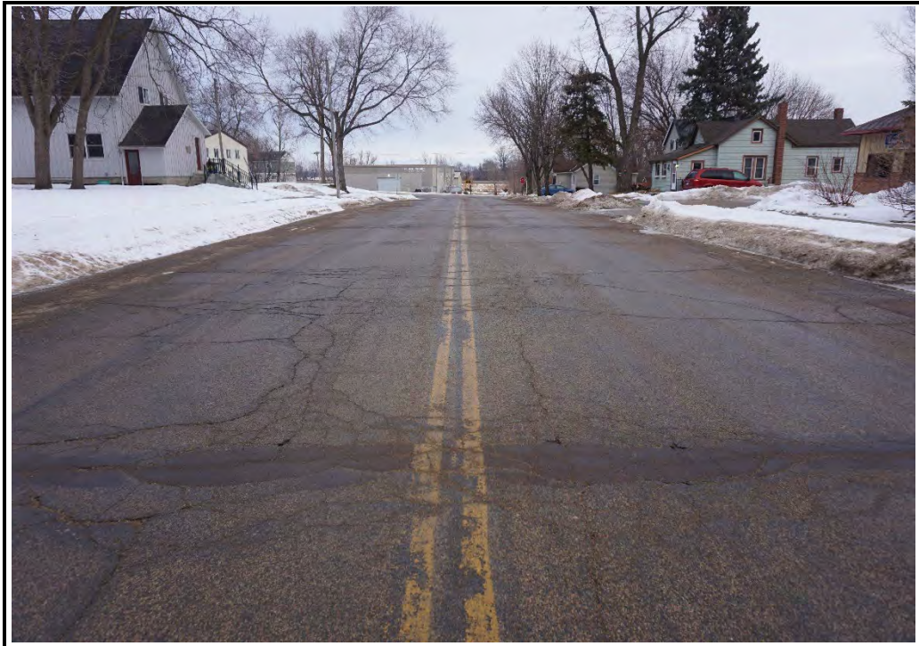
Looking North along N. Agency Street from adjacent to Duplex at 131-133 N. Agency Street
