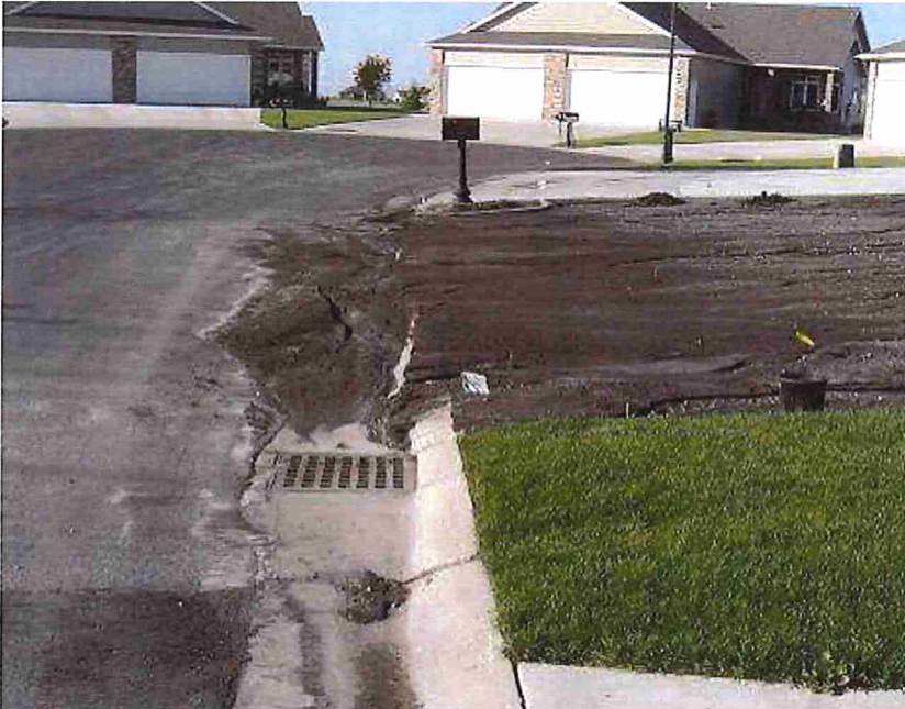
If no BMPs (ex. silt fence or silt fence w/ vegetation buffer), silt can run off and enter the storm sewer system as pictured left.
