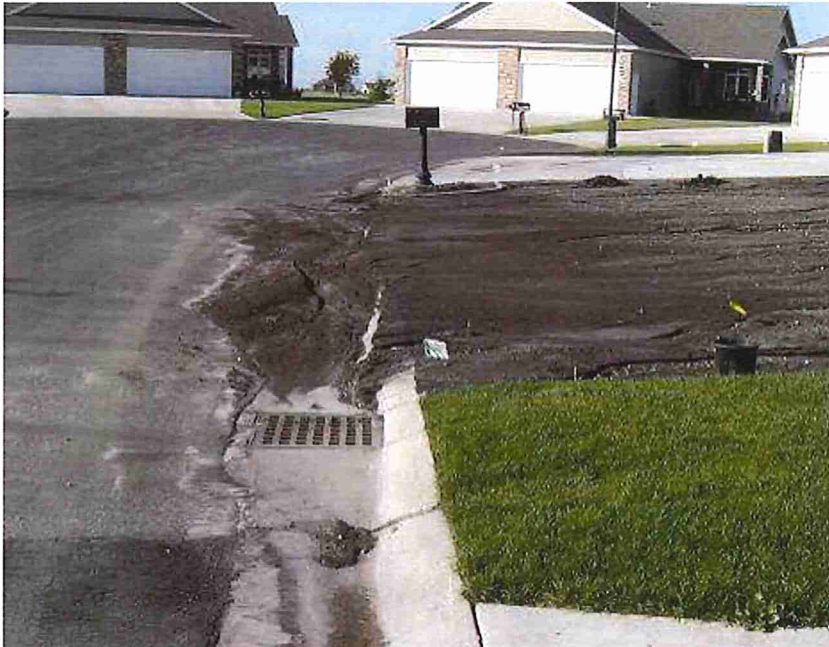
If no BMPs (ex. silt fence or silt fence w/ vegetation buffer), silt can run off and enter the storm sewer system as pictured left.
